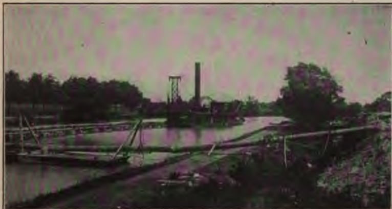
Discharge Pipe of Hydraulic Dredge. Figure 110.
